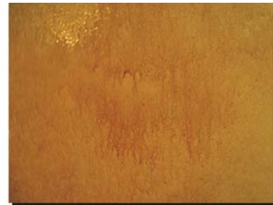
Platinum Wall Glazing Cream Drips in Damp Weather
